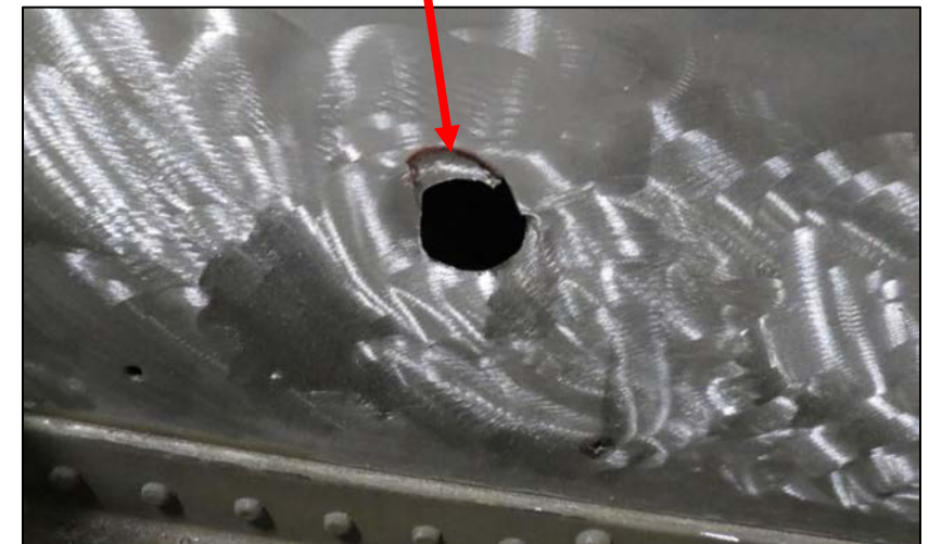
Damage Before Removal
