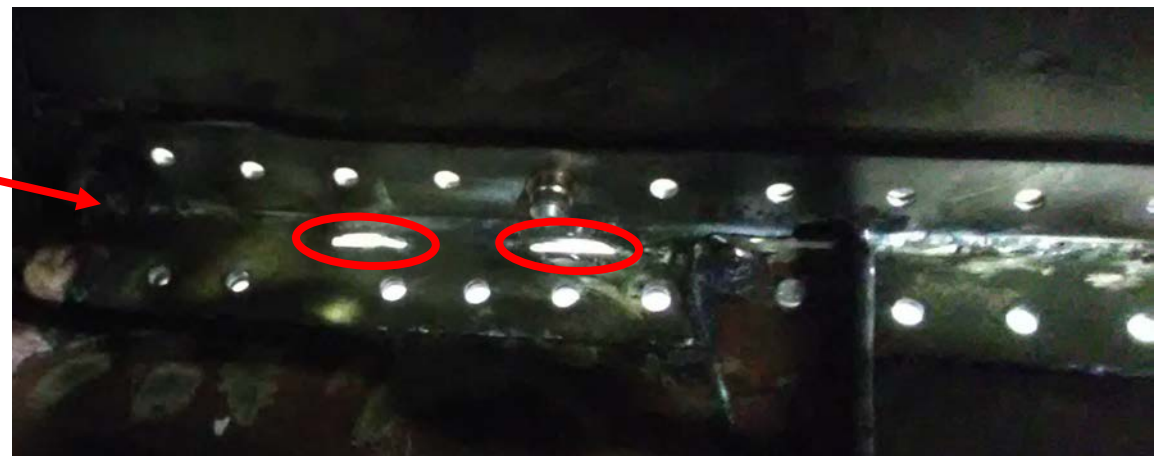
20Y Fitting (TOP), Closure Beam Corrosion (BOTTOM)
